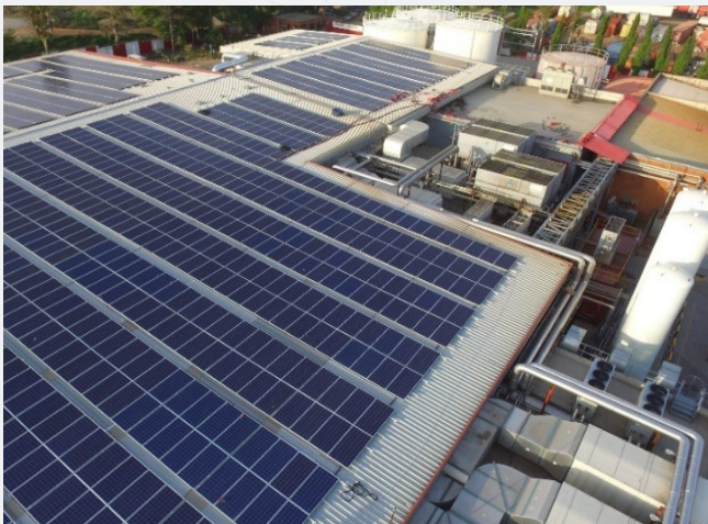
Exhibit 8. Rooftop solar system at NBC Abuja
